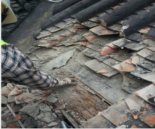
Rooftop in need of repair
